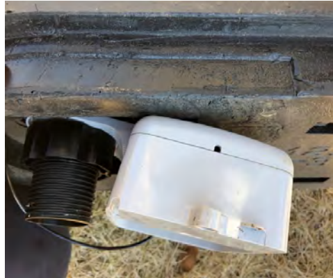
Figure 44 – Recessed Underside - Cellular Endpoint not Flush
