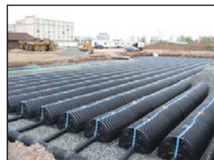
External conventional pipe and fitting manifold
