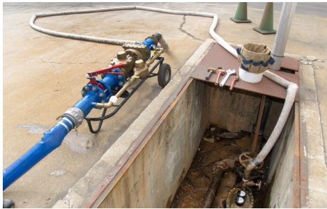
Figure 12 Filling the Test Equipment
