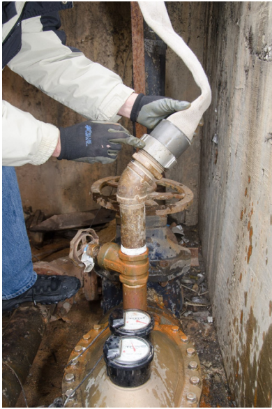
Figure 6 Connecting the Fire Hose
