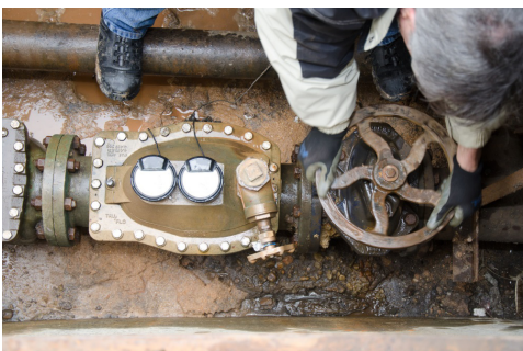
Figure 30 Isolation Valve - Downstream of Meter Under Test
