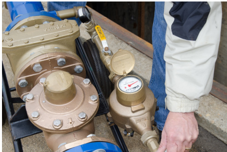
Figure 15 Open Reference Meter Outlet Valve
