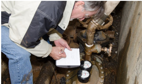
Figure 19 Meter Under Test Low Side Results
