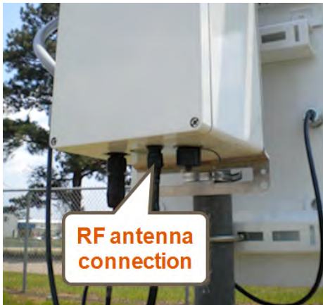
Figure 47 – RF Antenna Cable
