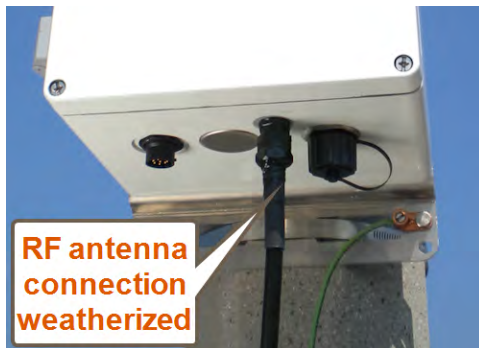
Figure 65 – Weatherized RF Port
