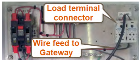
Figure 45 – Battery Box Wires
