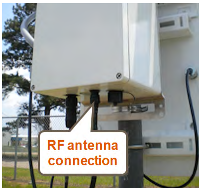
Figure 64 – RF Antenna Cable
