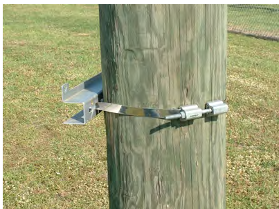
Figure 58 – Battery Box Clamps
