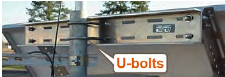
Figure 38 – Solar Panel Attached
