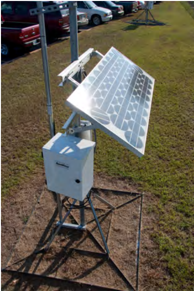
Figure 37 – Gateway Solar Panel
