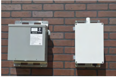
Figure 71 – UPS Mounted on a Wall
