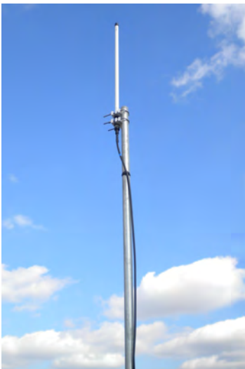
Figure 85 – Securing the Coax Cable
