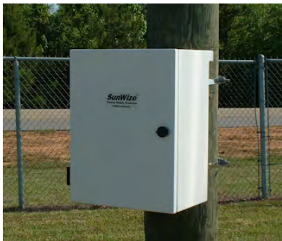
Figure 60 – Mounted Battery Box
