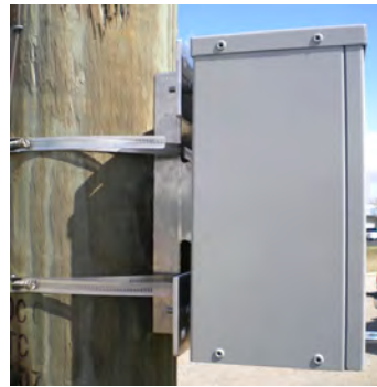
Figure 68 – UPS Attached with Clamps
