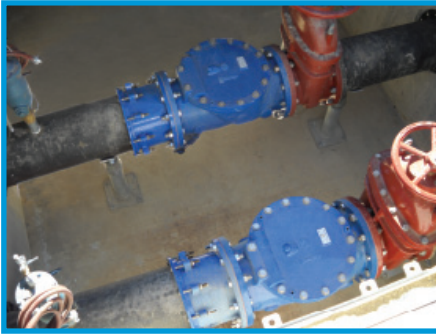
Swing-Flex® Check Valve installed in a Valve Vault
