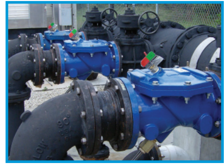
Swing-Flex® Check Valve with Mechanical Indicator installed in a Pump Station
